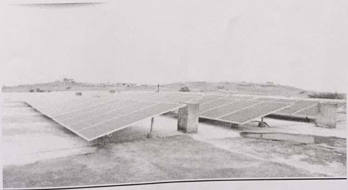
(Solar PV Roof Top 20 KW Net Metering System)
